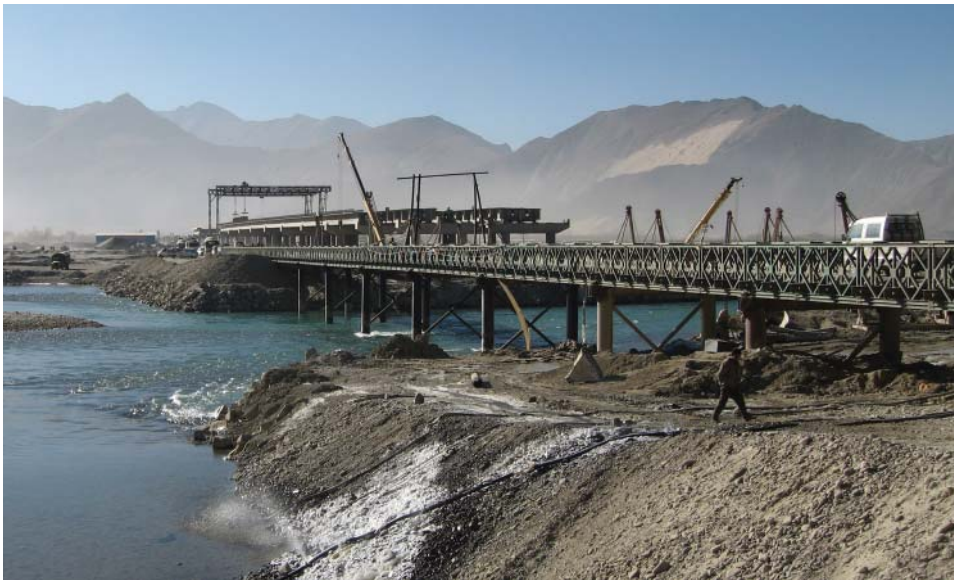
Work in progress on the bridge over the Kyichu River, to carry the road connecting the Chindrol Lam (Peaceful Liberation Road) with Lhasa station, January 2006.
