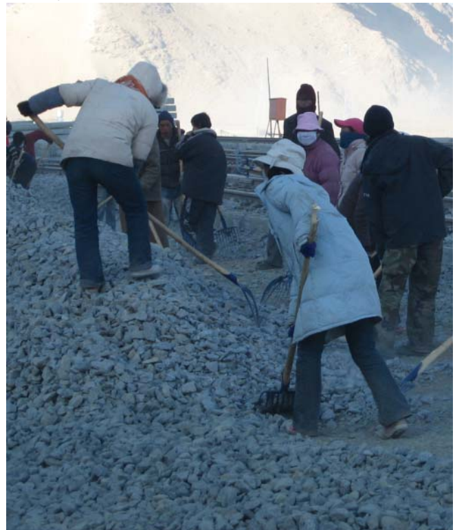
Workers toil on the tracks of the Lhasa railway near the station.
